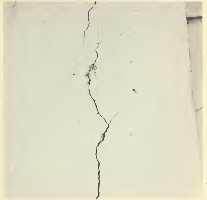
FIGURE 4. Popout around opaline shale fragment, Sixth Street Bridge, Los Angeles. Scale shown is 6 inches in length.
